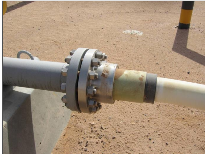
Figure 8: RTP Pipe coupled to a CS pipe via flange connection
